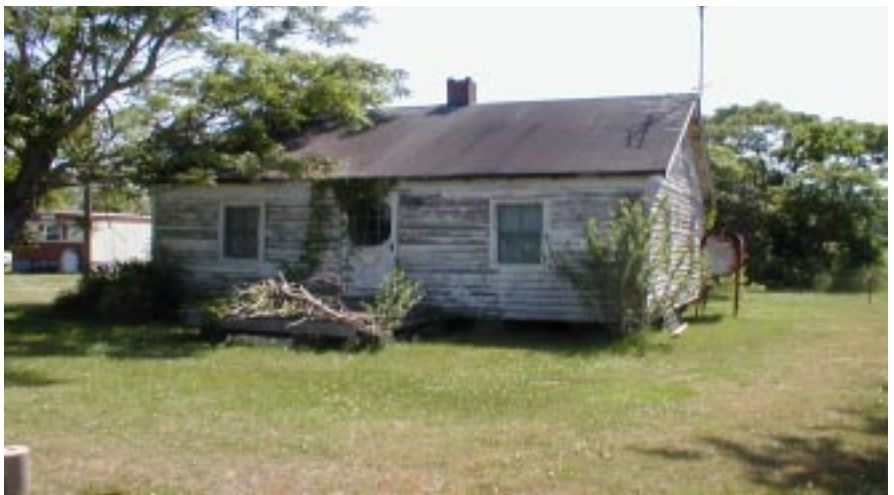
House lacking indoor plumbing
