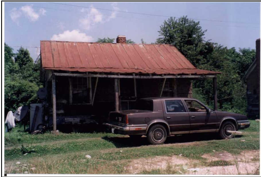
Deteriorated Housing Conditions on Woods Lane in Bayview
